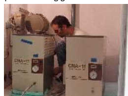
Figure 7 : Installation of the helium gas compressors to cool the iGravs
